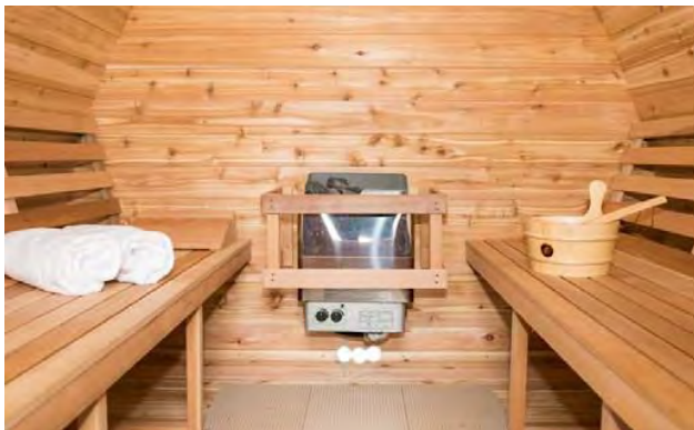
Inlet under electric heater on Back wall
