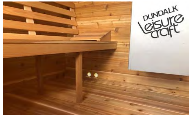
Inlet beside wood heater on Back wall
